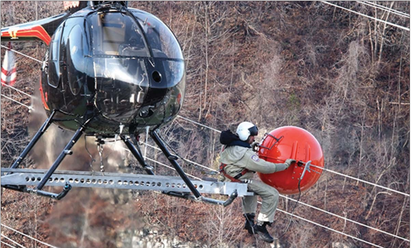
Above, a specially trained lineman performing marker ball replacement on a power line from a platform attached to a helicopter
