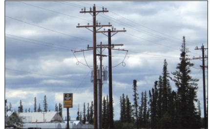
The Glennallen Double Circuit Project will improve reliability in the Copper Basin District
