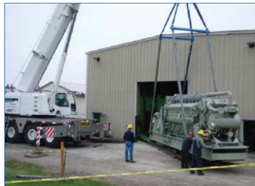
Glennallen Diesel Plant-Unit 9 Electromotive Diesel 2865KW
