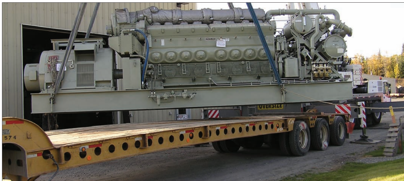
The EMD engine being offloaded and moved into its new home at the Glennallen Diesel Plant.
