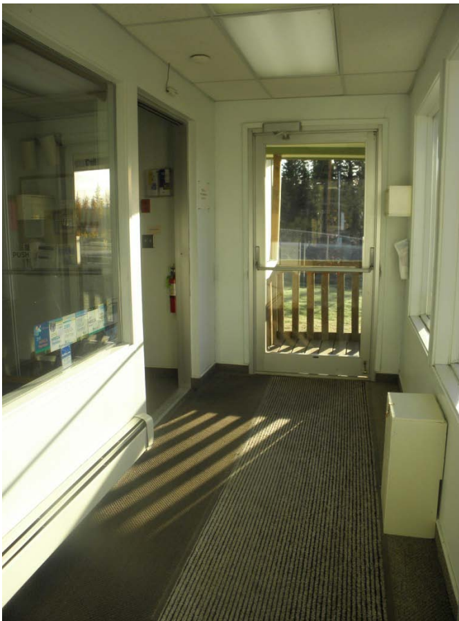
Existing Entry Porch-Needs Rebuilt or Updated
