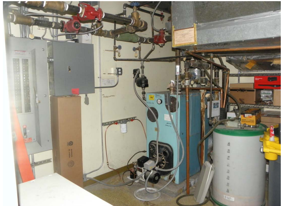
Boiler—Burnham PF35 – Need Replaced
