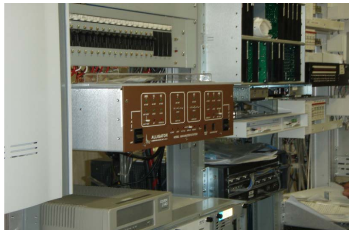
SCADA Master Radio
