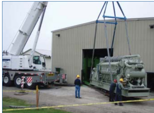
Glennallen Diesel Plant-Unit 9 Electromotive Diesel 2865KW
