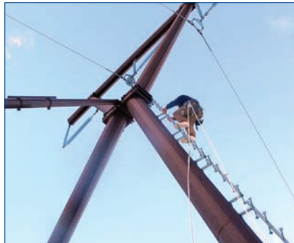
Glennallen Lineman, Ryan Cook, climbs a T-Line structure in Thompson Pass to make repairs
