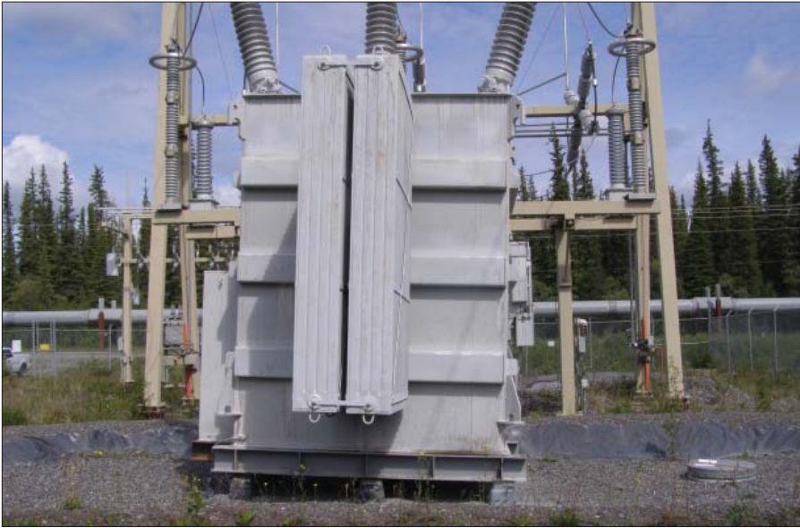
The CVEA Reactor at the Pump Station 11 Substation leaning from permafrost shifting its foundation.
