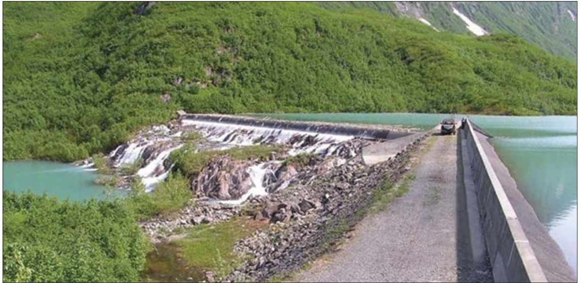
Solomon Lake Dike and Spillway; illustrates a full lake with water overtopping the spillway.
