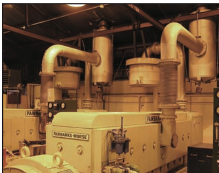
Glennallen Diesel Plant engines, installed in 1959; these engines will be replaced in 2009 after 50 yrs. of service
