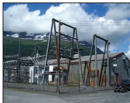
Valdez Diesel Plant and the Don Smith Substation
