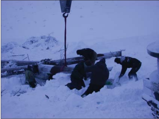
CVEA and City Electric crews getting the tower ready to be put back in place
